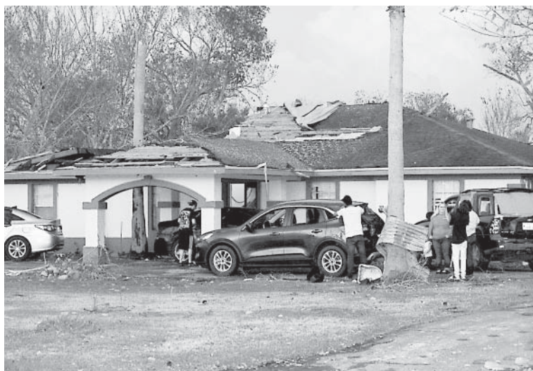
This photo shows a storm-damaged house near Walt Disney Elementary School in Alvin, Texas, the United States, December 28, 2024.
