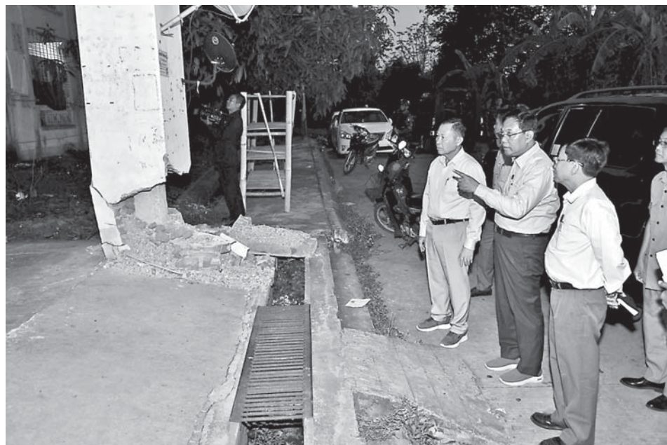
Vice-Senior General Soe Win inspects damage to Thazin Dormitory.
