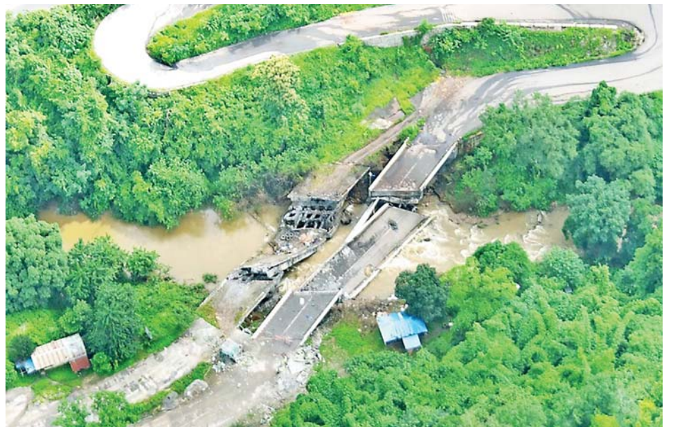
The photo shows the Goktwin bridge destroyed by terrorists.
