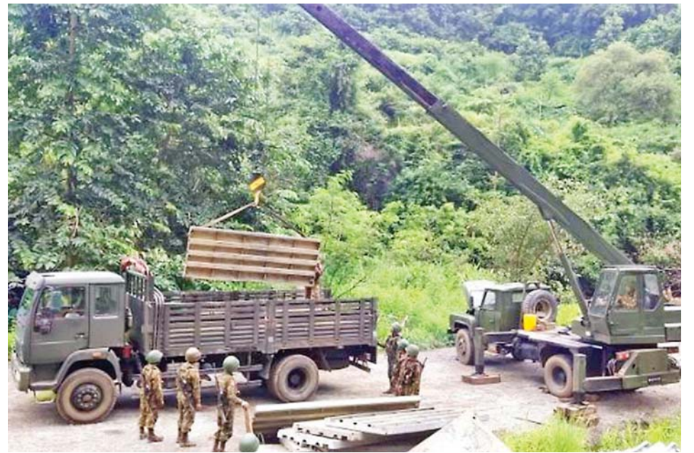
Tatmadawmen erecting a bailey bridge in the area near the destroyed Goktwin bridge.
