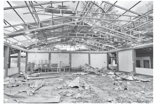
A school building destroyed by terrorist insurgents in Laykaykaw new town.
