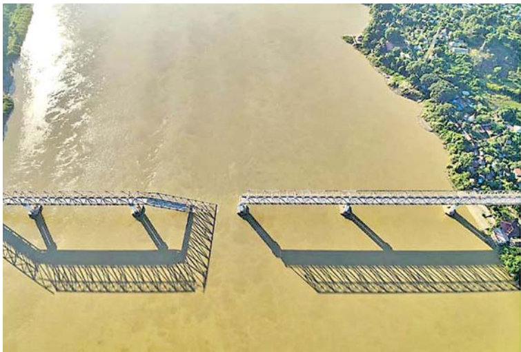
An aerial view of the Ayeyawady bridge (Yadanatheinkha), destroyed by PDF terrorist insurgents and collaborators.
