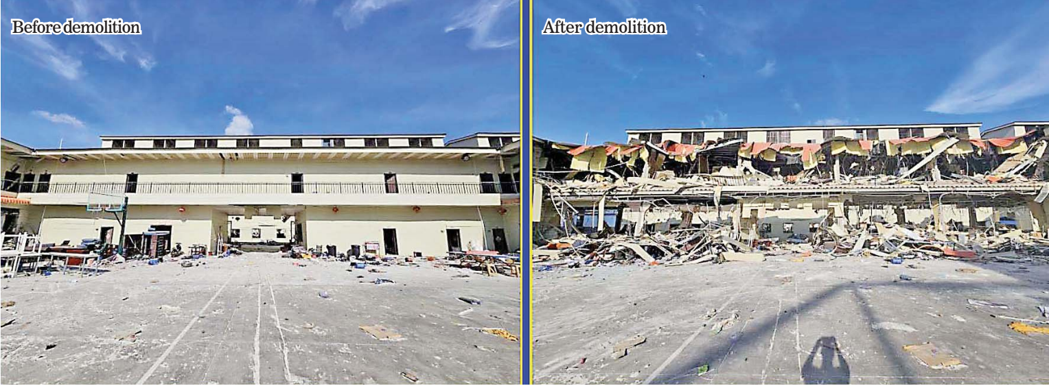
A documentary photograph showing a demolished two-storey building, which was illegally built in Part-3 of KK Park.
