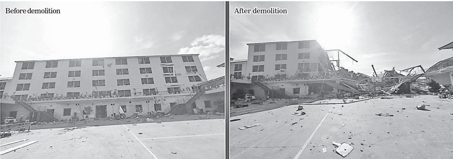
A documentary photograph showing a demolished five-storey residential building, which was illegally built in Part-3 of KK Park.
