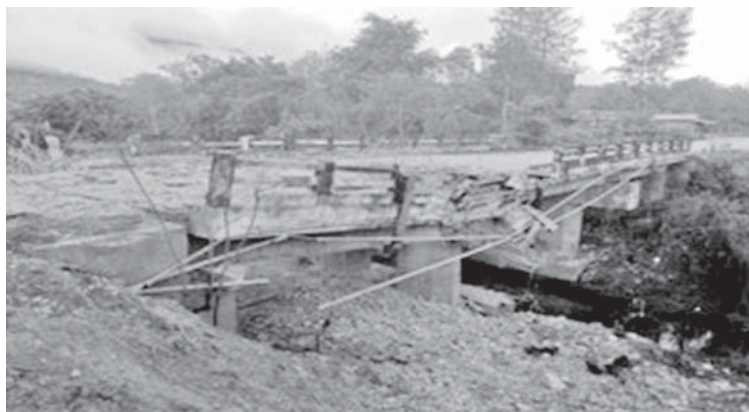
The destruction of Bridge No. 8 by planted mines during the temporary control by terrorist insurgent coalition groups.
